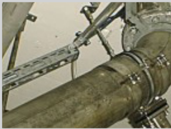
MARTIN® PKL® Interval Impactor 150 on transfer pipe
